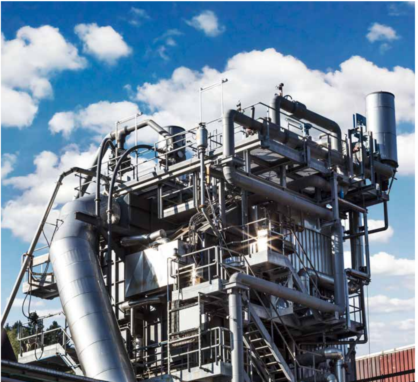
Heat Recovery Plant (IRC)
